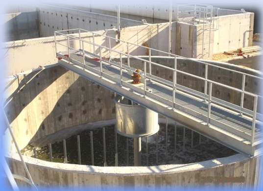
Thickener Bridge With Central Drive – PICC
