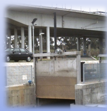
Motorized Penstock- PM
